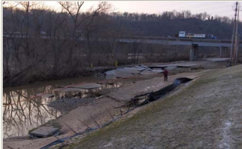
Figure 3: Damage to Yarnell Rd after the flood waters receded
