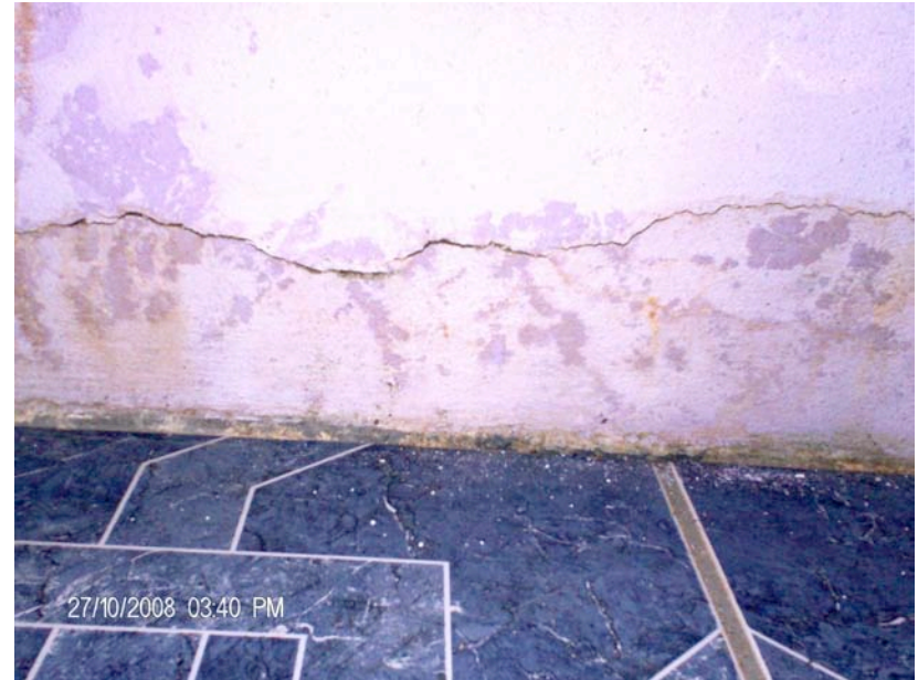
Figure 5d Type 4 Horizontal Crack
