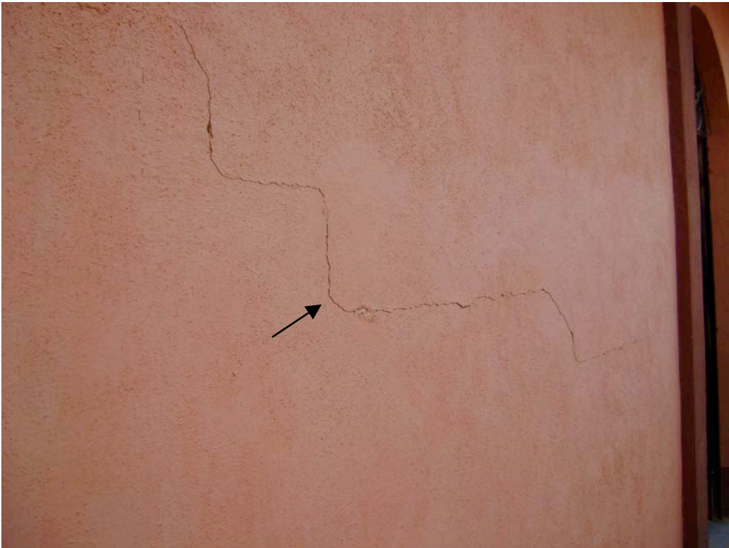
Figure 1d Crack in Concrete Block Grout
