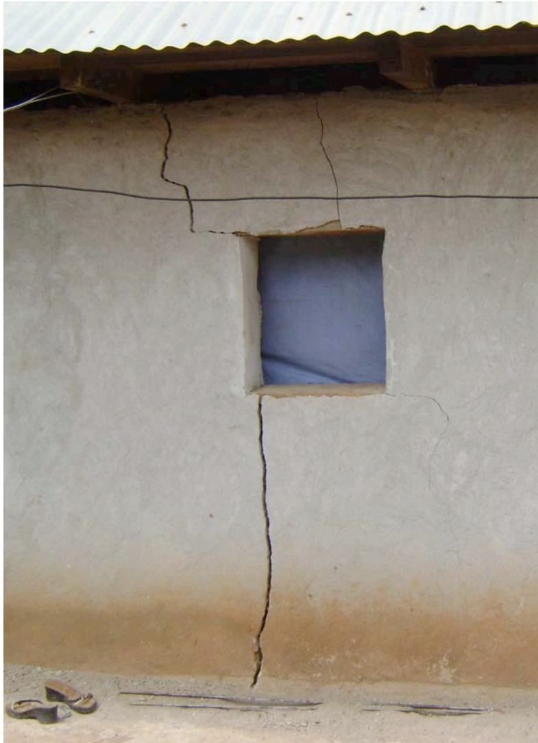
Figure 1a Vertical Wall Cracks in Adobe
