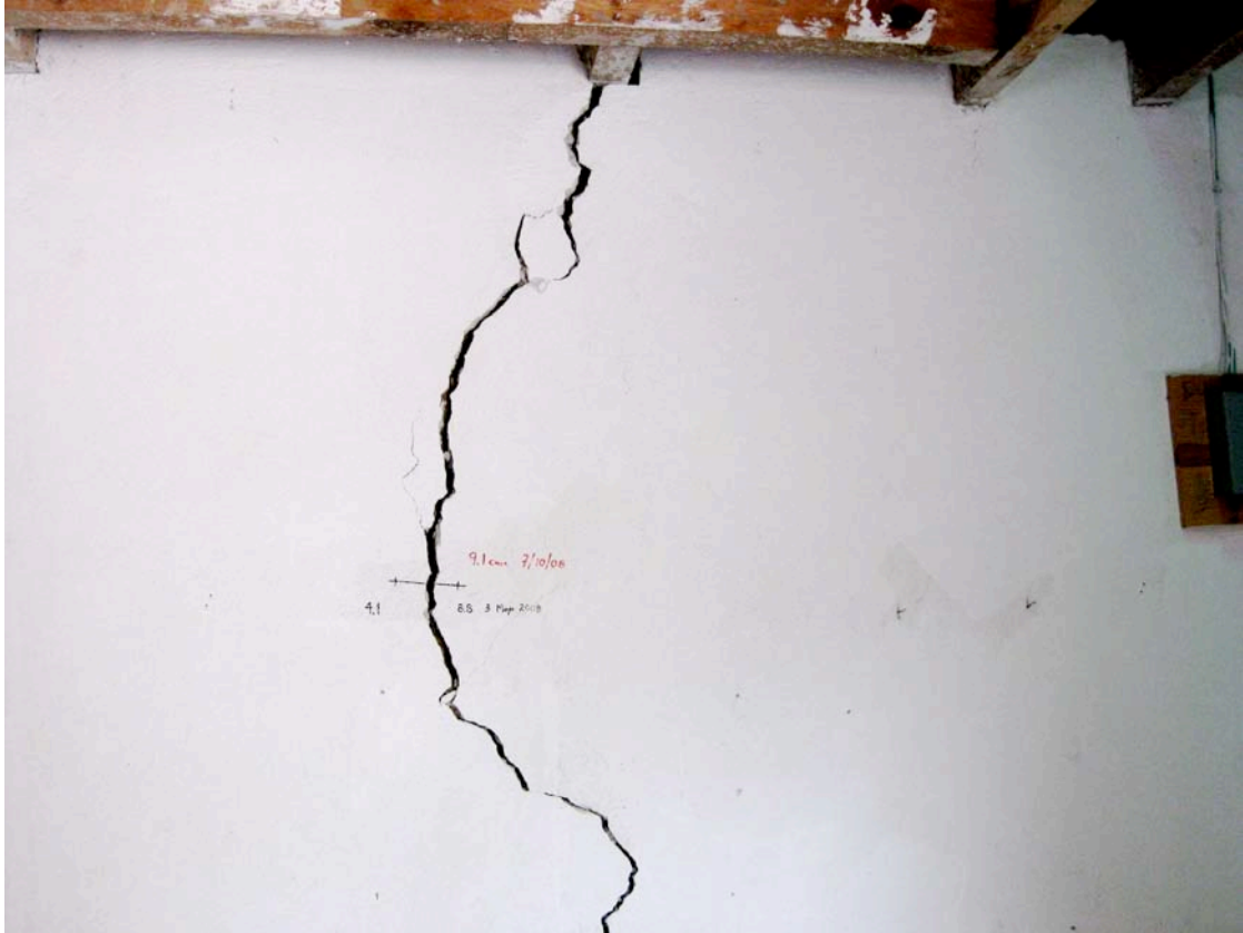
Figure 5e Type 5 Wall Crack Below Roof Beam
