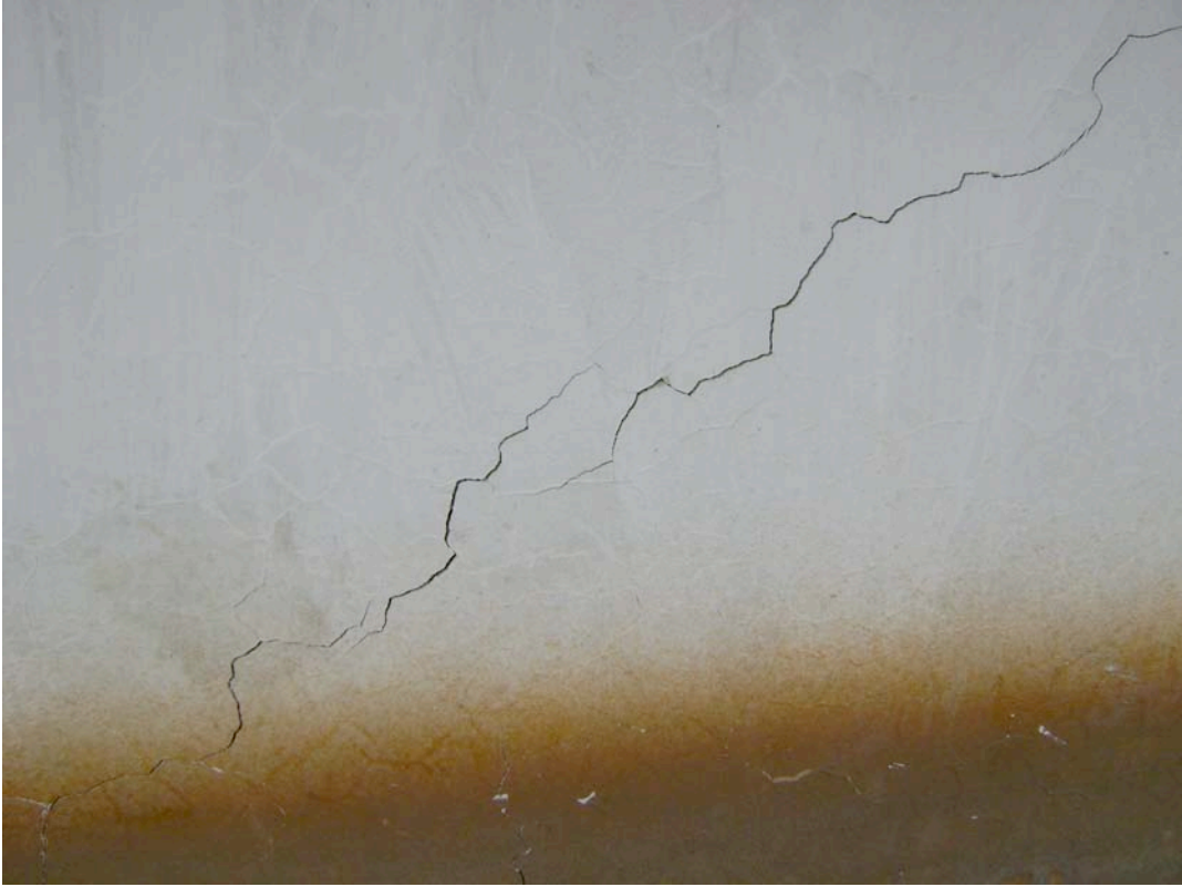
Figure 1c Incline Wall Crack in Adobe
