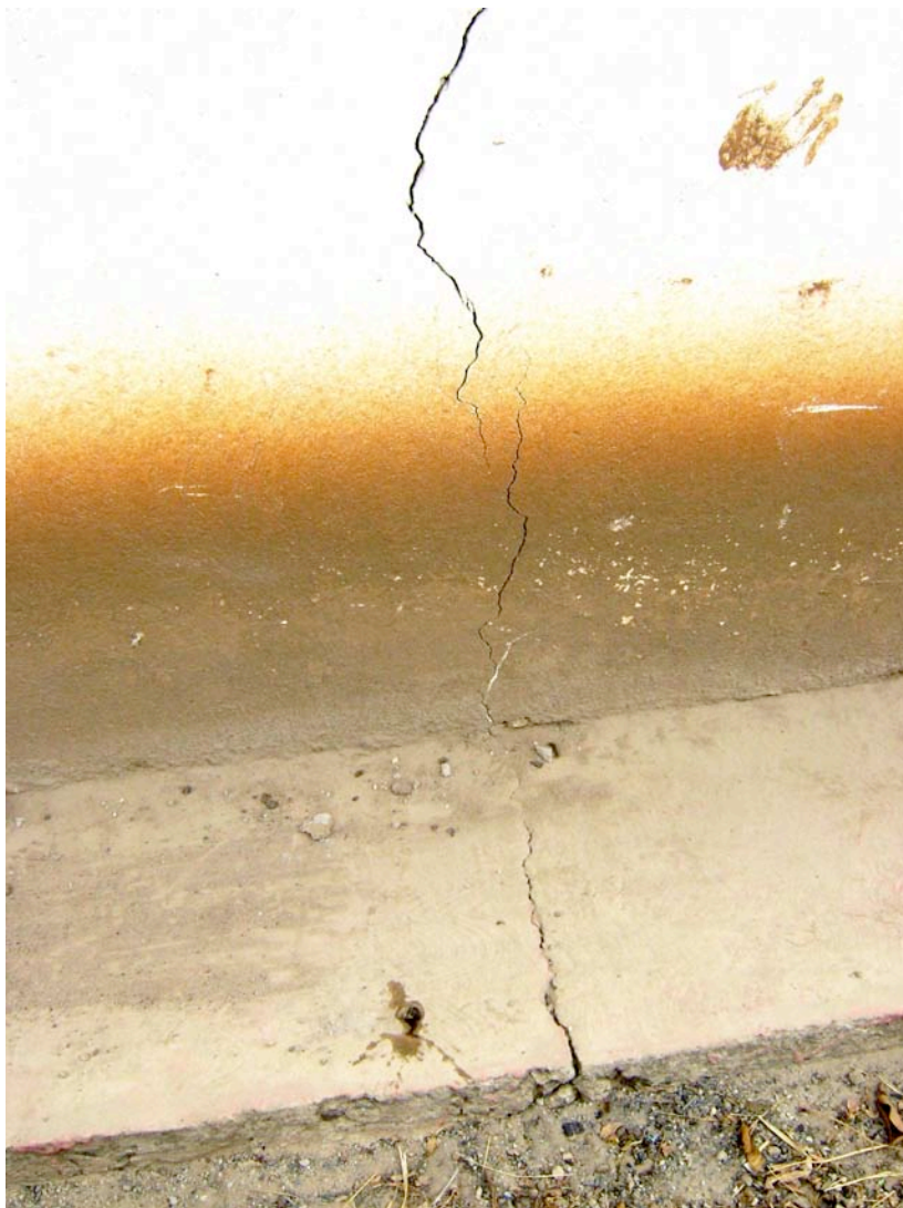
Figure 5c Type 3 Crack in Wall and Slab
