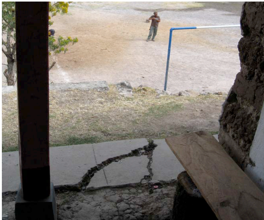
Figure 9b View From Building in Figure 9a (Fracture in foreground is same one shown in Figure 9a and it extends to person. Fracture difficult to see as it is partially filled with soil)
