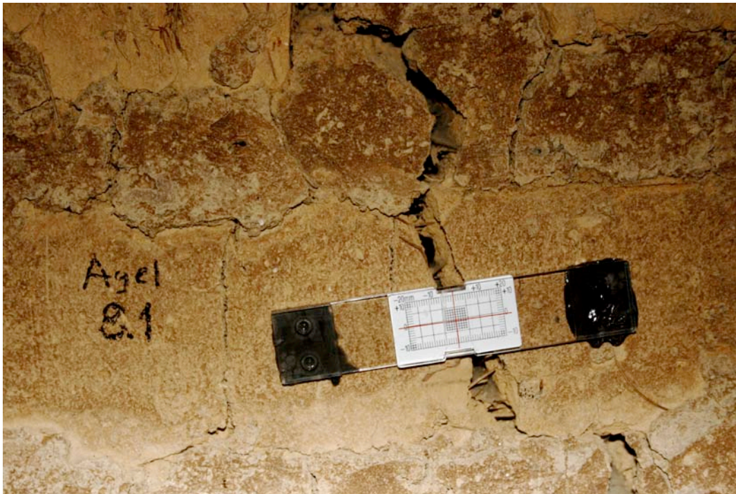
Figure 6b Crack Gauge
