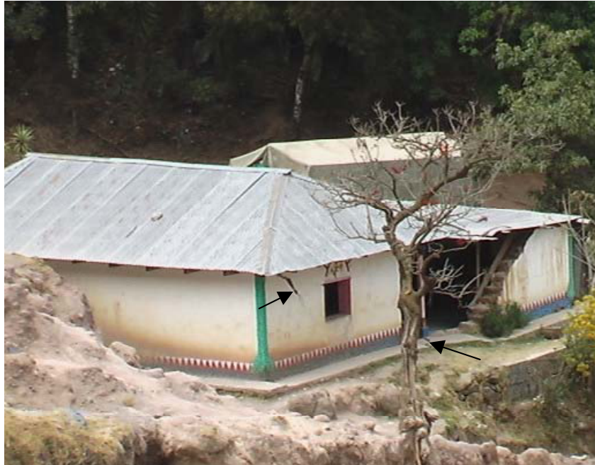
Figure 9a Damaged Building (note hole in wall, left arrow points to wall crack, right arrow points to fracture that extends into foreground)
