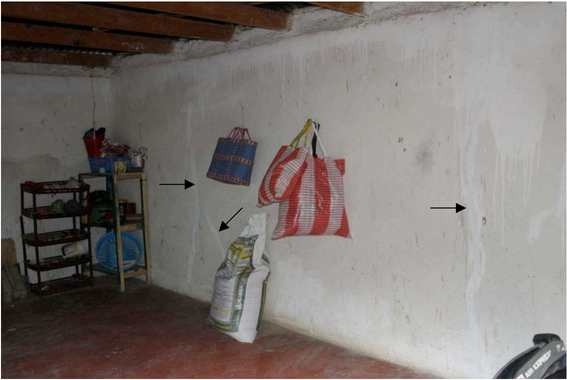
Figure 5a Type 1 Wall Cracks (3 covered with plaster), No Slab Cracks
