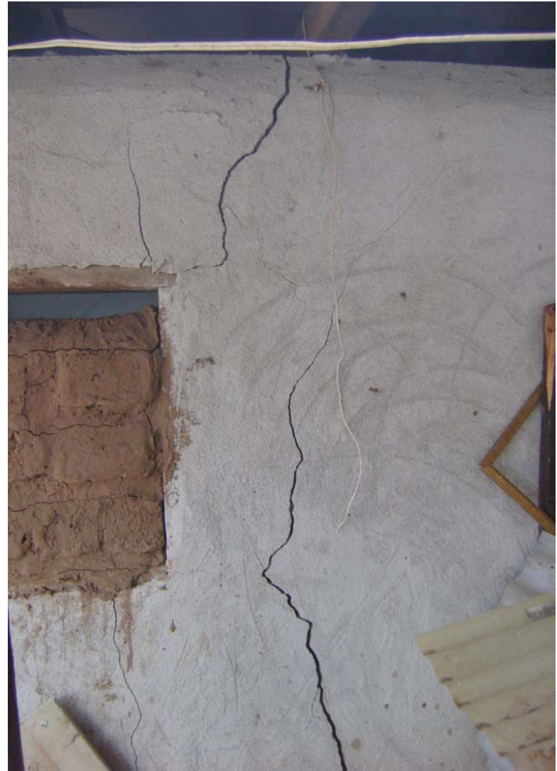
Figure 1b Vertical Wall Cracks in Adobe
